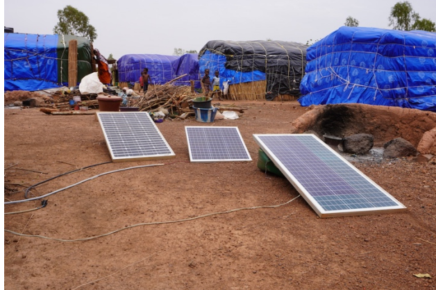
Picture: Solar energy in a camp of displaced people in Bamako, Mali. © Mirjam de Bruijn
